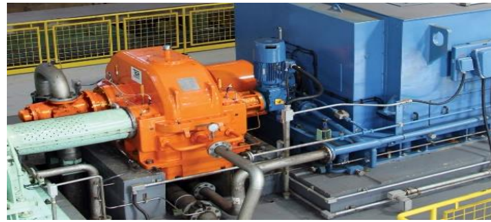
TGM Condensing Turbine Generator 30MW/11kV
