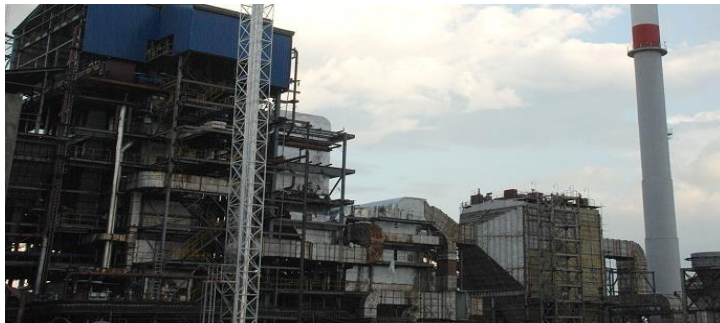
Boiler Pressure 40-70 Bar 140 ton/Hr
